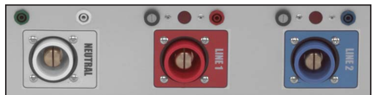
Above: Cam-Lok or MoleLock plugs with indicator lights and test jacks are included on all MolePower Pass-Thru Plus distribution boxes. (MoleLock not shown).
